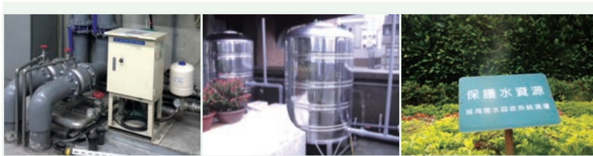
A gray water reclamation system was installed and a 1,296-ton rainwater reclamation tank was built in the headquarters basement to supply water for landscaping and toilets. In 2016, the gray water reclamation system helped conserve 16,610 metric tons of tap water, accounting for 7.9% of FFHC's total water consumption.
