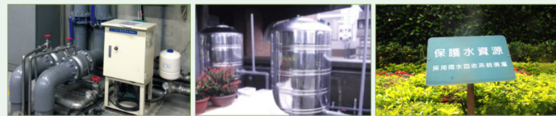
1 A gray water reclamation system was installed and a 1,296-ton rainwater reclamation tank was built in the headquarters basement to supply water for landscaping and toilets. In 2017, the gray water reclamation system helped conserve 33,757 MT of tap water, accounting for 14.5% of the FFHC's total water consumption.
