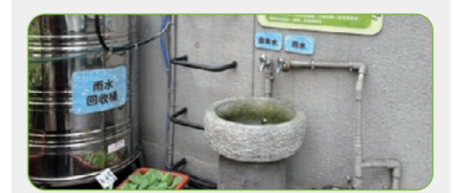
Rainwater harvesting system at the Wanhua Branch
