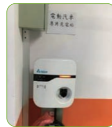
EV charging stations have been stilled at our Zhongli Branch and the Yanping Building, which are complete with dedicated charging equipment for EVs
